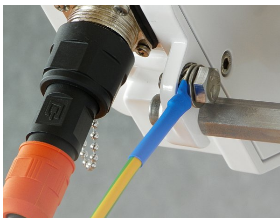
Fig. 5.67: Protective conductor at the FOD unit
